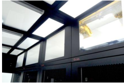
Cabinet supported roof
